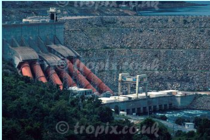
Electricity generating station at base of dam wall; huge pipes carry water past it from Lake Volta. Akasombo Dam, Ghana
